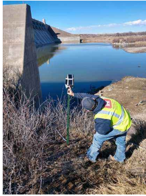
Figure 9: John Martin employee installing flood sensor downstream of the dam.
